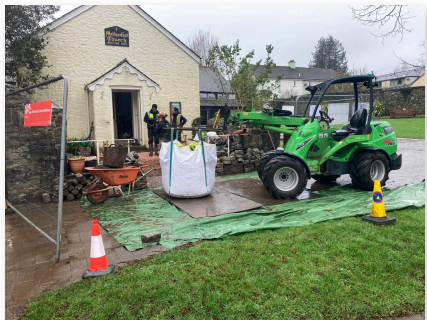
Contractors, Unique Projects at work on the front approach to Buckfast Chapel
